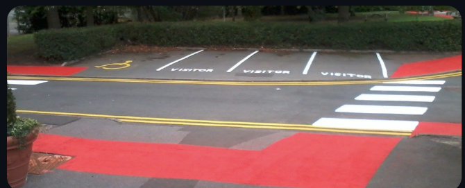
epoxy resin & thermoplastic markings
